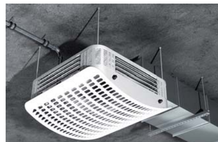
Air conditioning units
