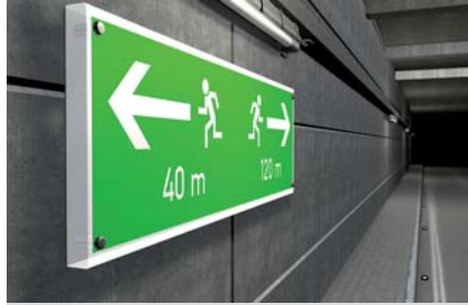
Emergency exit signs in tunnels
