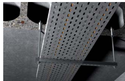
Cable trays in pre-stressed hollow-core concrete
