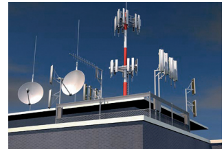
Antenna and masts
