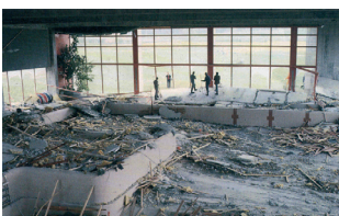
In 1985, the suspended concrete ceiling of an indoor swimming pool collapsed in Uster, Switzerland. The stainless steel ceiling attachments exhibited no external defects, but were completely destroyed internally in some cases due to stress corrosion cracking.
