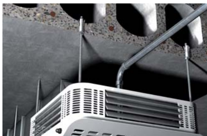
Air conditioning units in pre-stressed hollow-core concrete slabs
