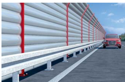
Crash barriers and sound insulation walls
